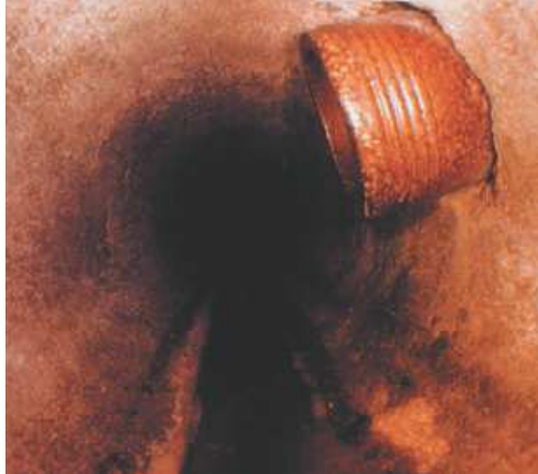
Damaged side inlet – inward projecting pipe socket
