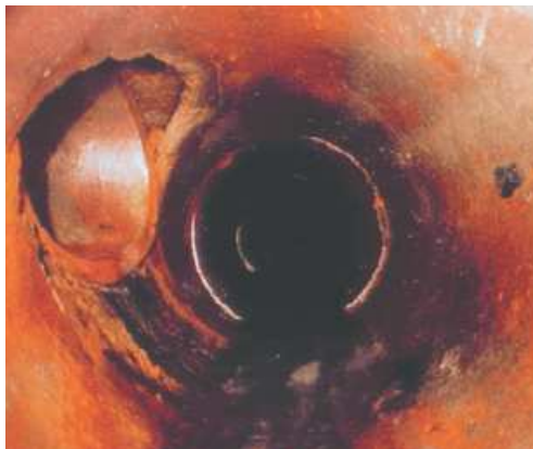
Damaged side inlet
